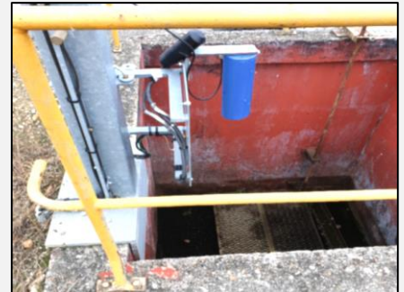
Sump water monitoring
