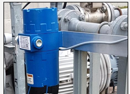
HazLoc area monitoring
