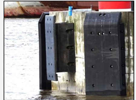
Fixed port installation
