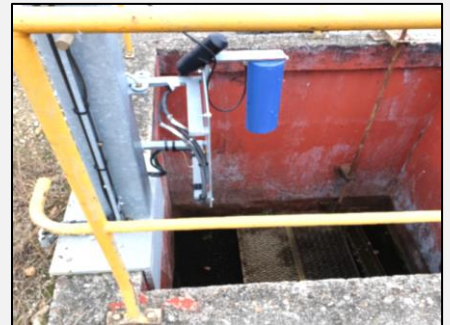
Stormwater, process, plant & cooling water monitoring
